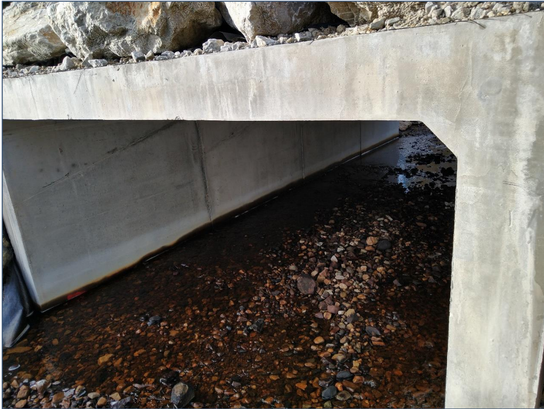
Plate 4-13 Example of an existing concrete box culvert crossing along the proposed access route
